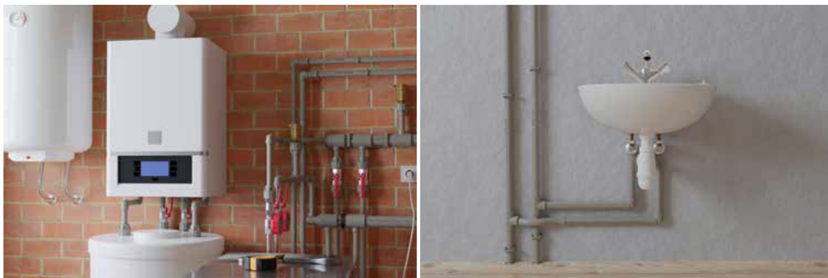
KAN-therm PP installations
