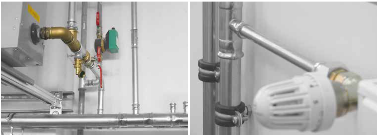
Examples of KAN-therm Steel installations
